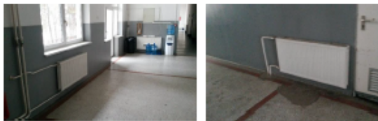
Figure 12 – Radiators installed in the building
