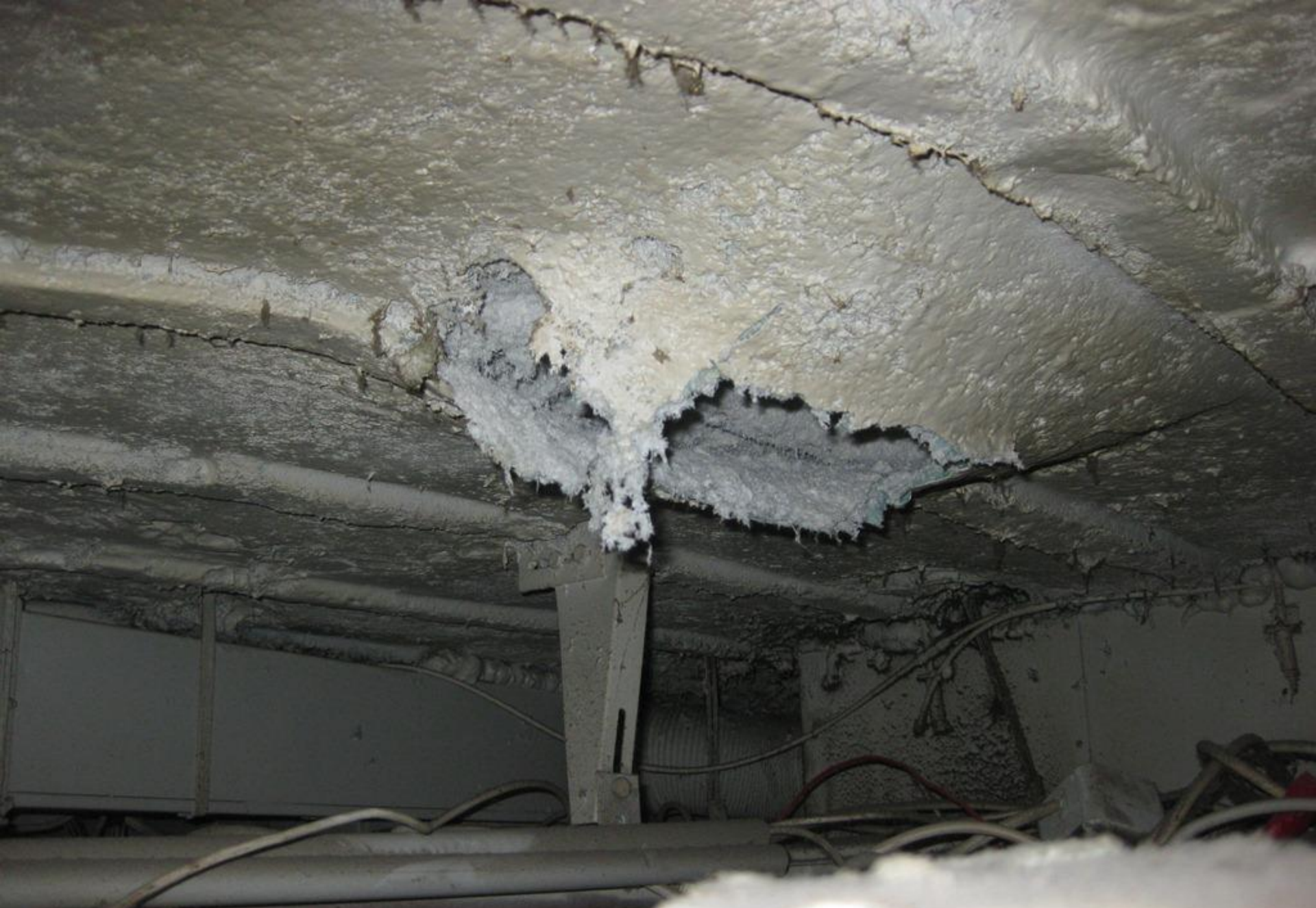
Sprayed asbestos cement(fire protection) metal ceiling/BS- Spritzasbest Metalldecke (4)
